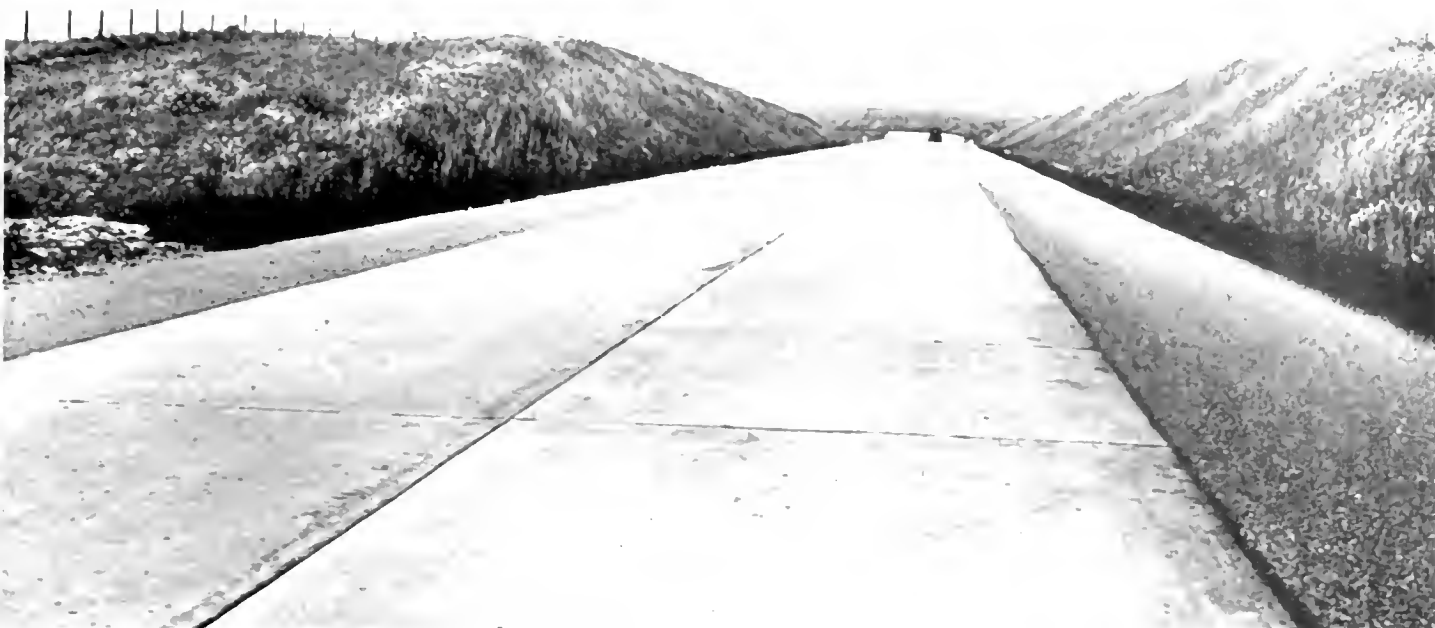
Completed 2-lane Portland cement concrete pavement between Marina and Castroville. Paved gutters and erosion protection on slopes show in this picture
